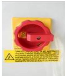
Picture 7 – Main switch OFF
