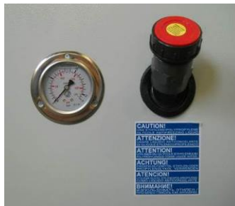
Picture 9 – Example of filling point
