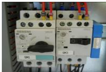
Picture 8 – Circuit breakers OFF
