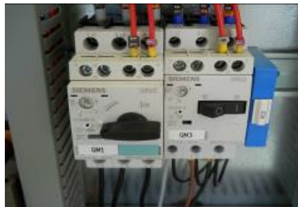
Picture 15 – pump breaker On
