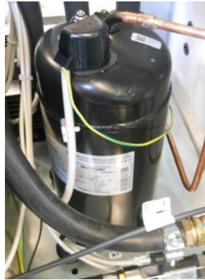
Picture 21 – Compressor placement
