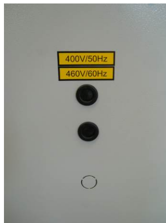
Picture 13 – Electrical connections
