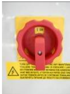
Picture 16 – Main switch ON
