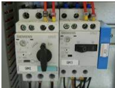
Picture 19 – All circuit brakers ON
