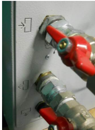
Picture 12 – Pipe connection
